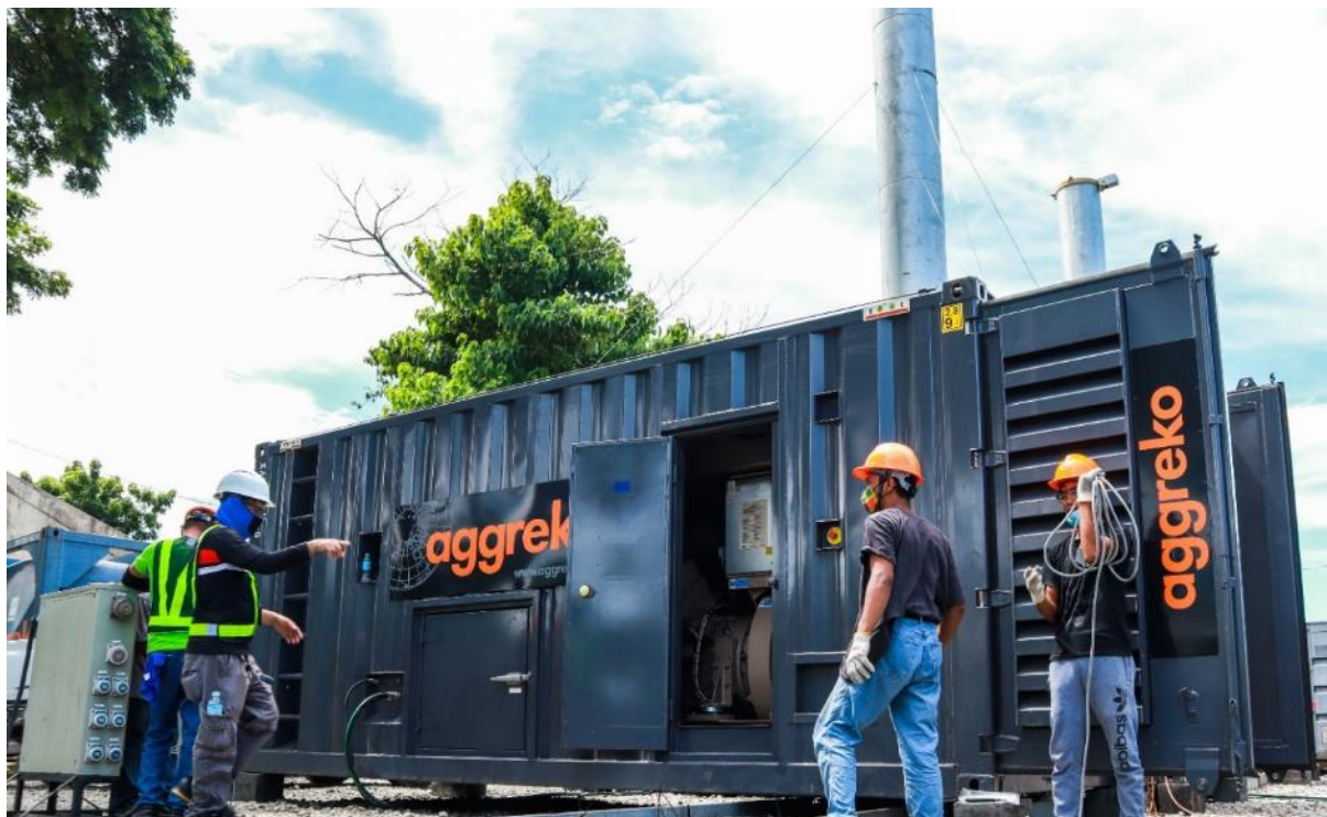
INEC installed generators with a combined capacity of 3 megawatts to provide emergency power to BANELCO’s franchise area.
