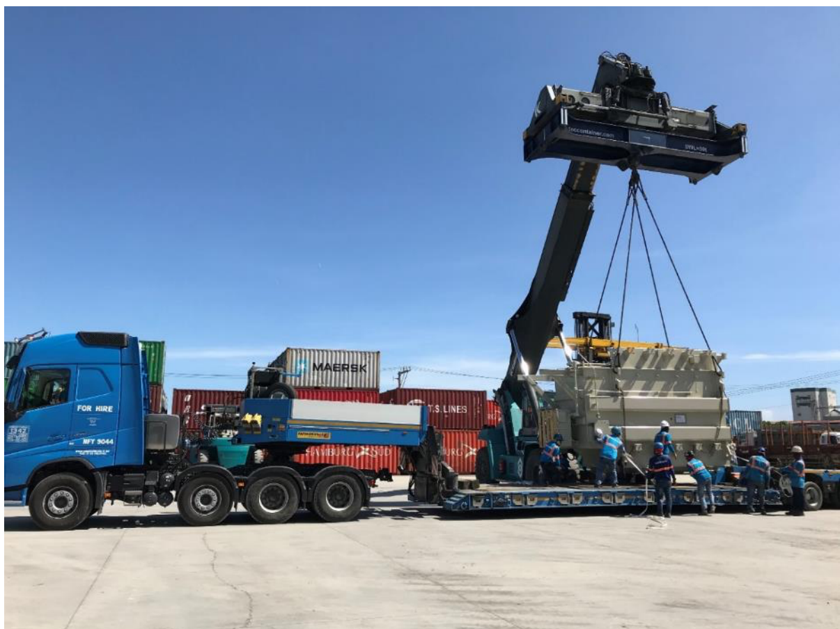
The transformers and related equipment for the 23.3-MW Isla Norte Energy Corporation power plant were delivered to Bantayan in November 2020.
